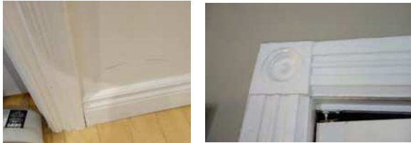
There is a very limited amount of 19 th or early-20 th century millwork in some areas on the first and second floor.
