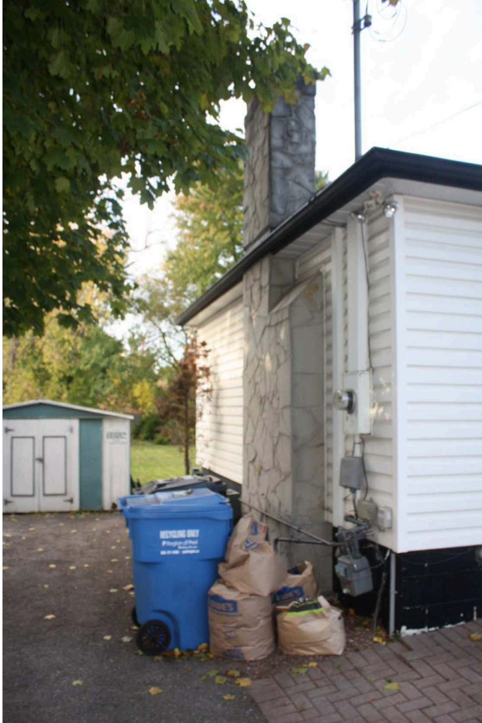
Figure 17 The south façade of 70 Queen Street South showing what is likely a replacement fireplace chimney. The utility shed is partially visible at the rear of the house. (Photo by author, October 2018.)
