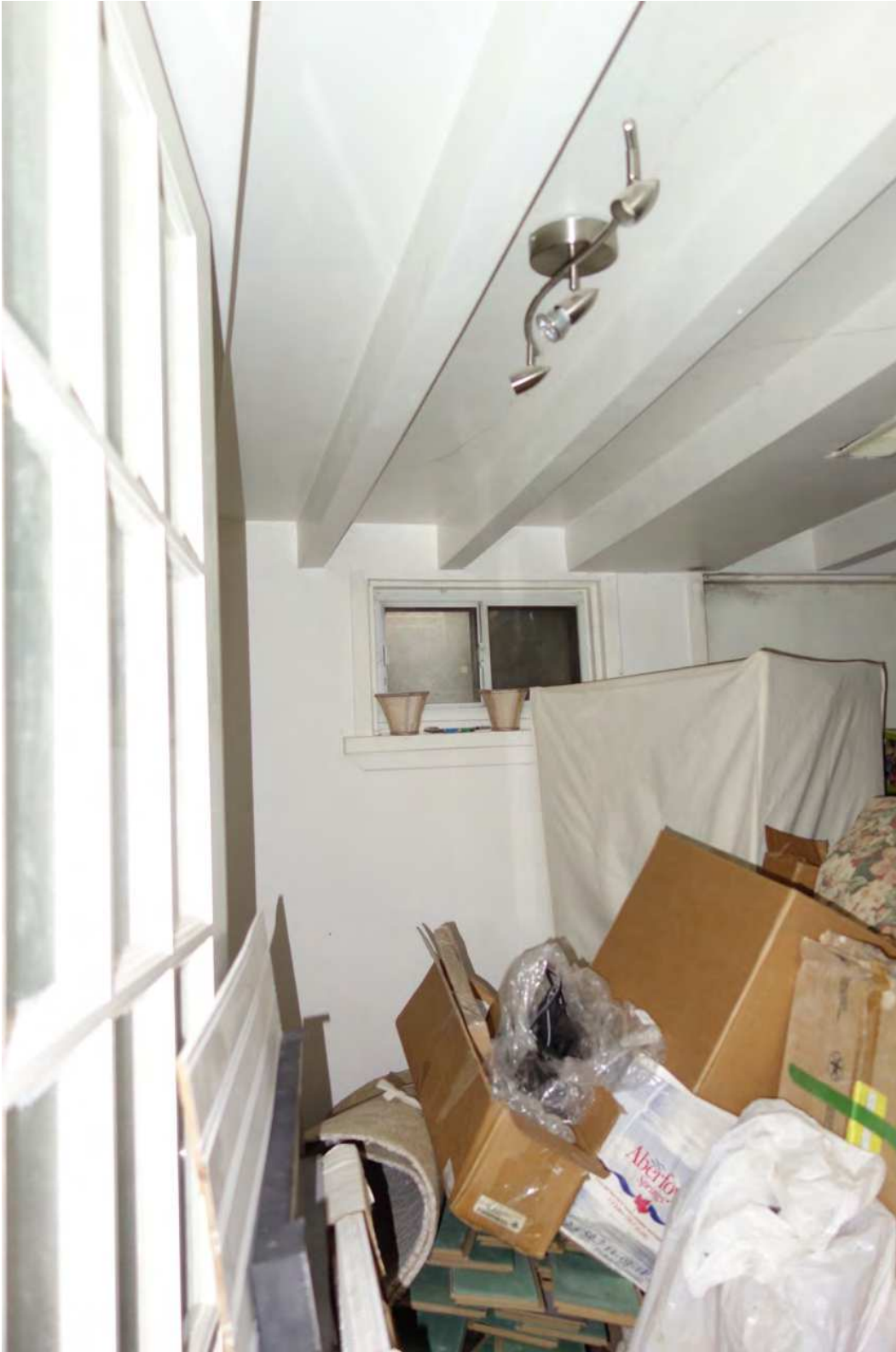
Figure 43: 24 Ann Street - INTERIOR - BASEMENT - storage room - exposed beams with modern spray stucco finish - modern window
