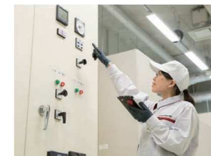
Daily facilities checks
