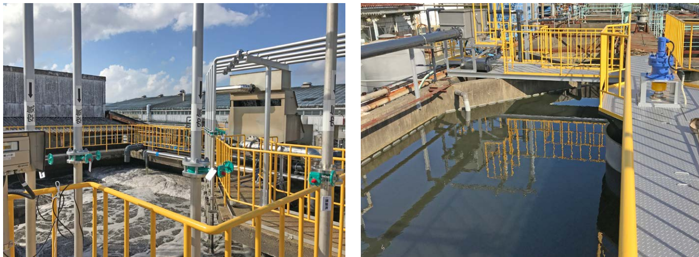
Sekisui Nano Coat Technology wastewater treatment facility
