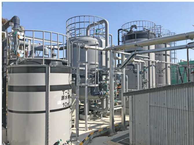
Water filtration equipment at the Shiga-Minakuchi Plant
