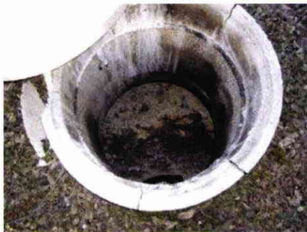
Concrete riser breaking down from the corrosive effects of an anaerobic septic tank
