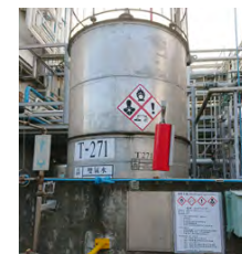
GHS labeling on a storage tank (example)
