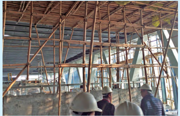
施工現場02(珠海学院新校舎) Construction site 02 (Chu Hai College of Higher Education new building)
