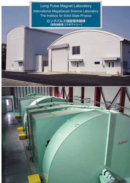
Fig. 2. The building for the flywheel generator (left hand side) and a long pulse magnet station (right hand side). The flywheel giant DC generator is 350 ton in weight and 5 m high (bottom). The generator, capable of a 51 MW output power with the energy storage 210 MJ, is planned to energize the long pulse magnet generating 100 T without destruction.
