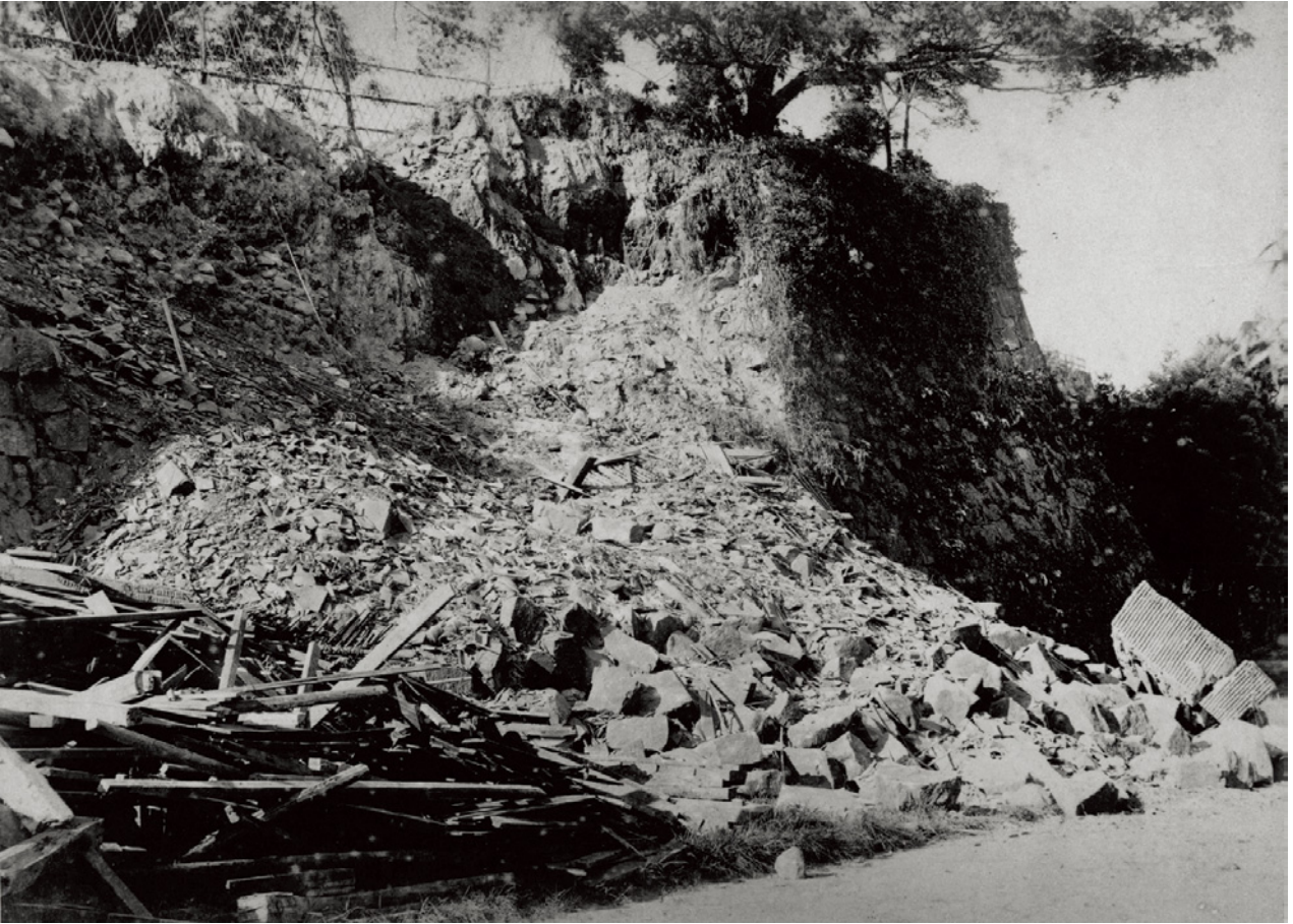
図 4 旧熊本城西出丸 第六師団火薬庫崩壊之景(国立科学博物館蔵). Fig. 4 A photograph of damaged 6th Division Gumpowder at Nishidemaru (owned by National Museum of Nature and Science)
