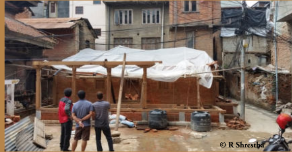
Community of Om Bahal is rebuilding its heritage with support from Nepal Government and technical support from KVPT. Newar craftsmen & community play a pivotal role in rebuilding. Date:- July 28 2019
