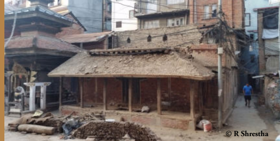
This is an ancient 200 years old community building & rest house called Om Bahal sattal located in Patan city. This building was heavily damaged after 2015 earthquake in Nepal. Date:- May 13 2019
