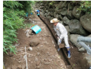
Removal of sediment from waterways in Kurogi, Yame city, Fukuoka in 2012' flood disaster.
