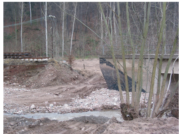
Photo 2 Railway damaged by flood with sediment
