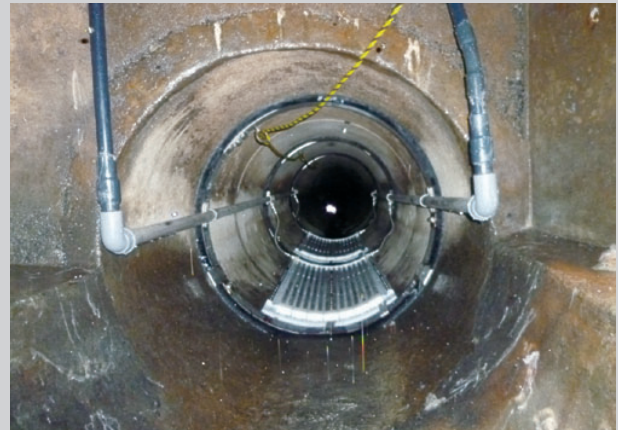
下水熱蓄熱融雪システムの開発に関する研究(管底設置型金属製熱交換器) Research on development melting system of snow, using wastewater heat reserve (a metal heat exchanger installed at pipe bottom)
