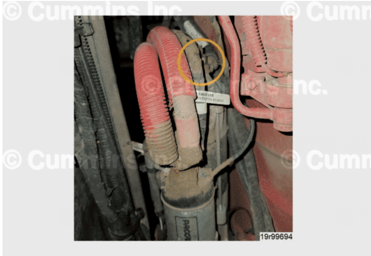
Figure 1, Location of Loose Power Return (Ground) Connection at Starter that Resulted in Fault Code 2349.
