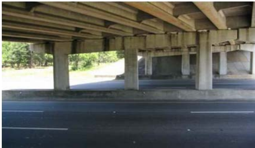
Photo 8: Staining on sides of pier caps
