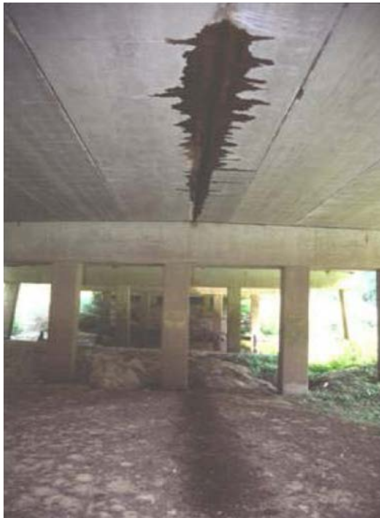
Photo 6: Staining along longitudinal joint. Note guano deposits on the ground.
