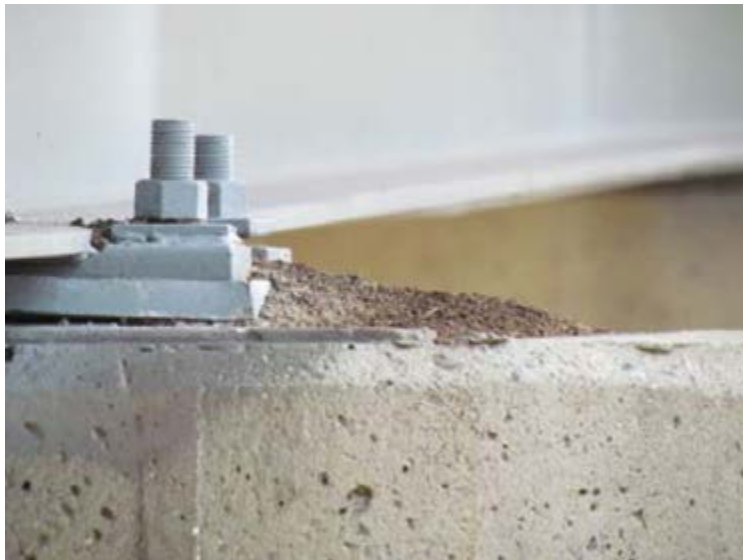
Photo 4: Guano deposit on pier, obscuring structural features
