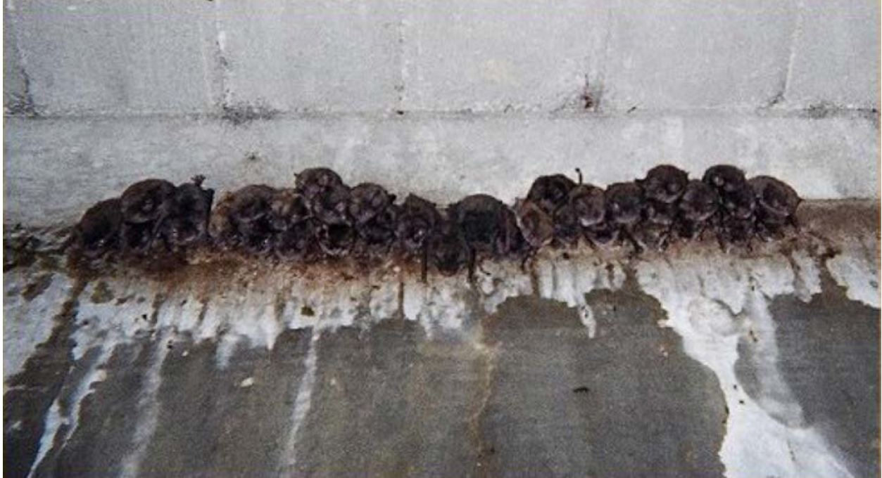
Photo 9: Bats roosting and associated staining
