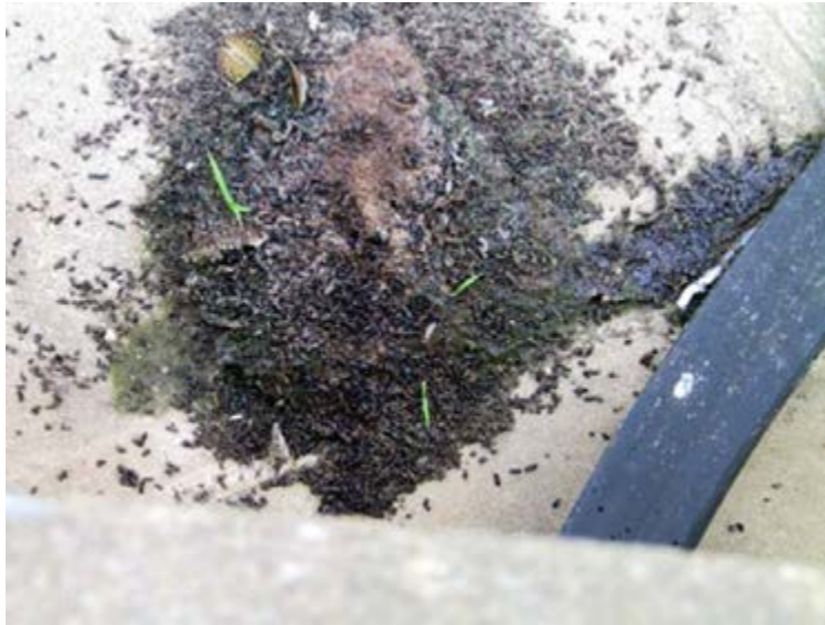
Photo 3: Guano deposits visible from bridge deck, on top of pier
