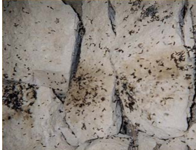
Photo 5: Bat guano on rip rap
