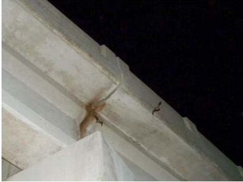
Photo 7: Staining on underside of expansion joint from bat use
