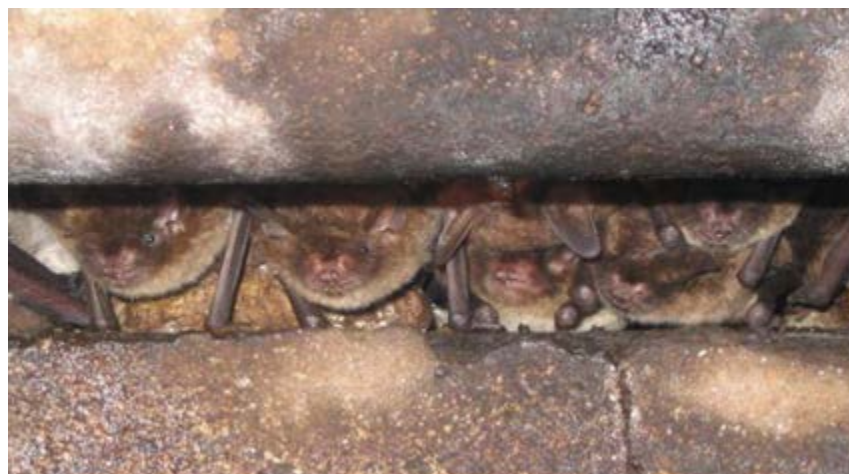
Photo 2: Visible bats within an expansion joint
