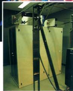
A view towards the loop cabinets sited behind the projectors.
