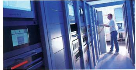
Partial view of the control and source racks. They include a CCTV system to monitor the Core Show.
