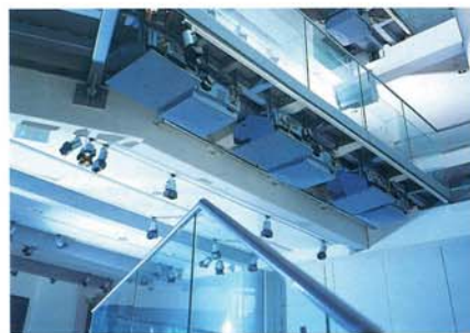
A view of the projectors, mounted under the foyer balconies. Notice how some projectors are inverted to get them nearer the screen centre line. Photo from Barco.
