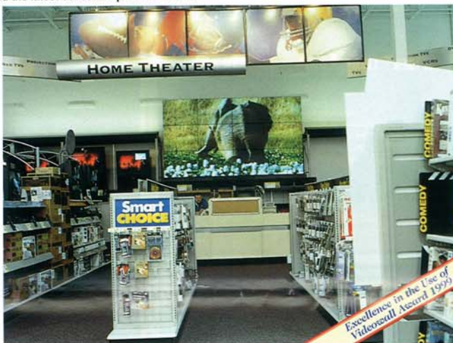
One of 90 Electrosonic High Definition Videowalls installed at Best Buy locations throughout the USA.
