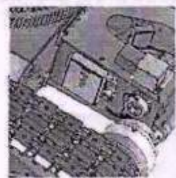
Lower control cabinet
