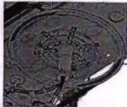
MV collector rings on the revolving frame
