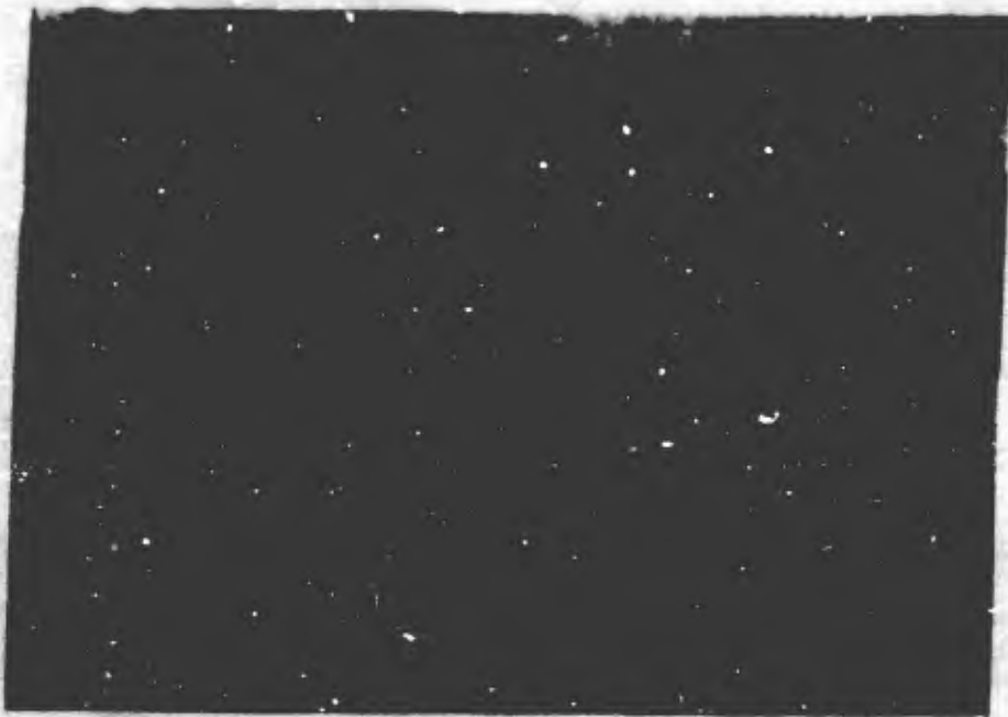
Figure 139. Crack and settling in the concrete floor of the Anadyr' fish cannery. The rulers show the amount of settling of the floor of the building. Photo by S. P. Kachurin.
