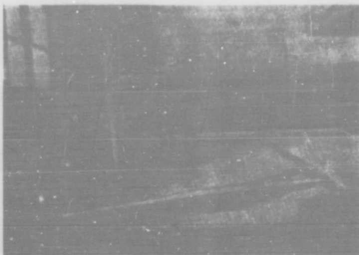
Figure 139. Crack and settling in the concrete floor of the Anadyr' fish cannery. The rulers show the amount of settling of the floor of the building. Photo by S. P. Kachurin.
