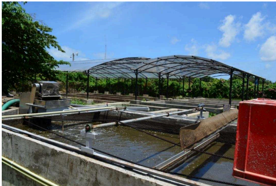
Figure 6: Treating wastewater in a small-scale plant in Colombo Municipal Area
