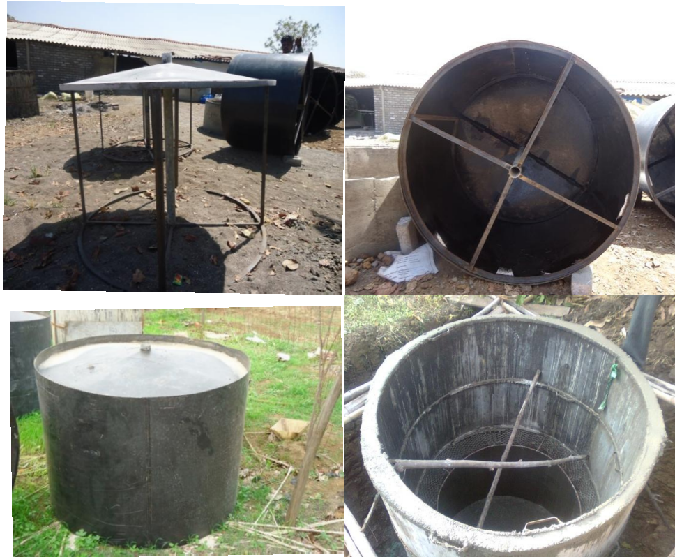
Figure 3.1 Different components of the digester tank
