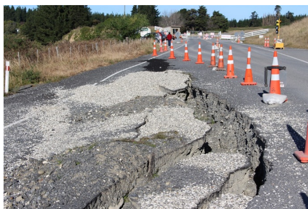
Figure 2-2 Cracks in the road
