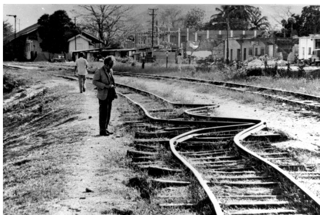
Figure 2-5 Damages to railway rails during Tangshan Earthquake
