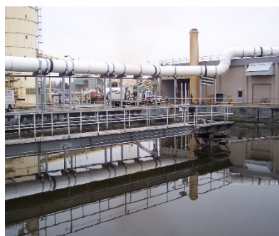
Figure 2-7 Water supply station
